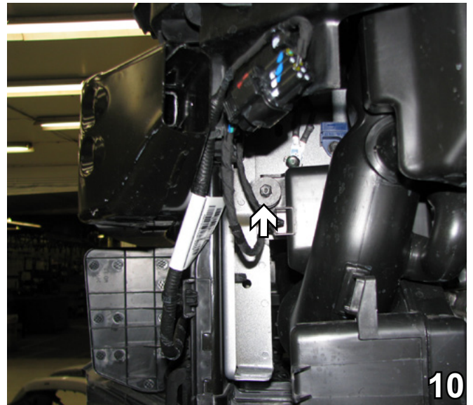
10. On the driver side, using a 10MM socket remove the one (1) bolt on the outside of the air baffle.
